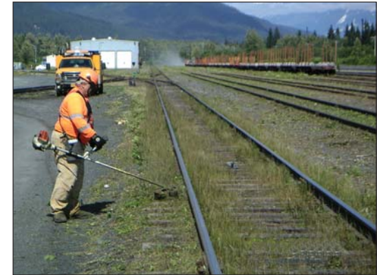
Ineffective mechanical / manual vegetation control in the Seward Yard prior to herbicide application.
