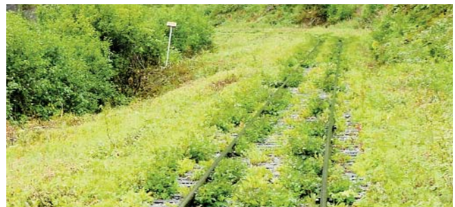
Overgrown weeds on the track bed are nearly impossible to get rid of with non-chemical methods.
