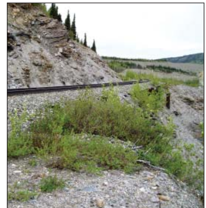
The existing retaining wall at MP 357 is deteriorating. Track needs to be realigned away from the Nenana River.
