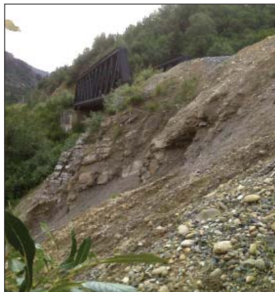
A retaining wall needs to be installed at MP 355.2.
