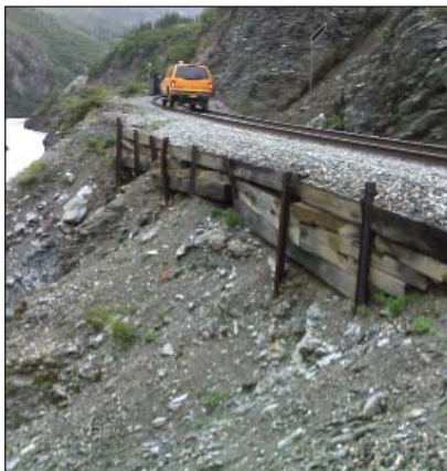
The track bed retaining wall at MP 354.1 needs to be replaced.
