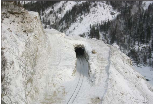
2008: Moody Tunnel is prepped for the final step in a series of demolition steps to remove the top from the tunnel.
