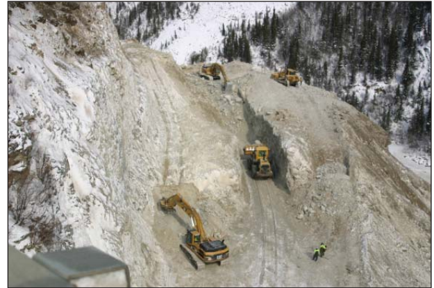
Crews clear debris after a demolition explosion April 17, 2008. Moody Tunnel daylighting was completed in 2009.
