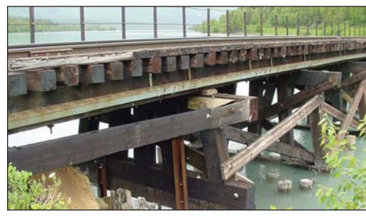
Timber piling and caps were replaced with steel pipe and pile caps on the bridge at MP 29.5 in 2011. In 2012, timber beams and ties will be replaced.
