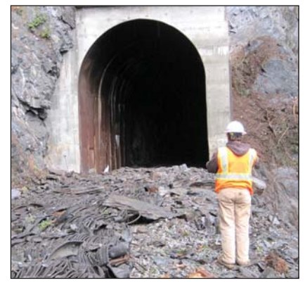
At the opening of the tunnel near MP 52, rubber tire pieces protect the rail as debris falls due to recent scaling operations to remove loose rock. A more permanent solution is a rock shed.
