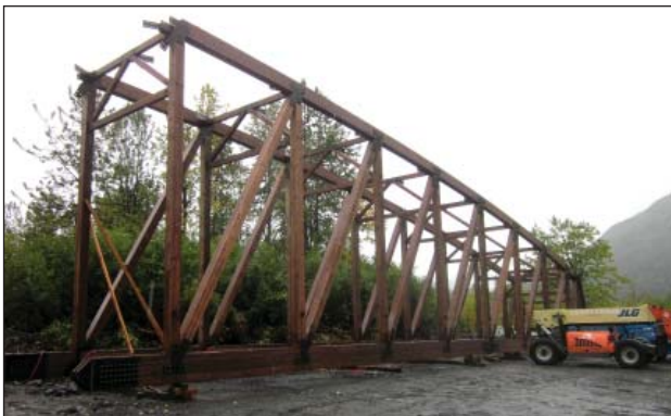
Construction on the first of two pedestrian bridges began in summer 2011. It will allow trail users to cross the Placer River.
