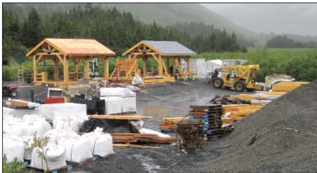
Construction gets underway on the Grandview Whistle Stop site in summer 2011. Construction is due to resume in summer 2012.
