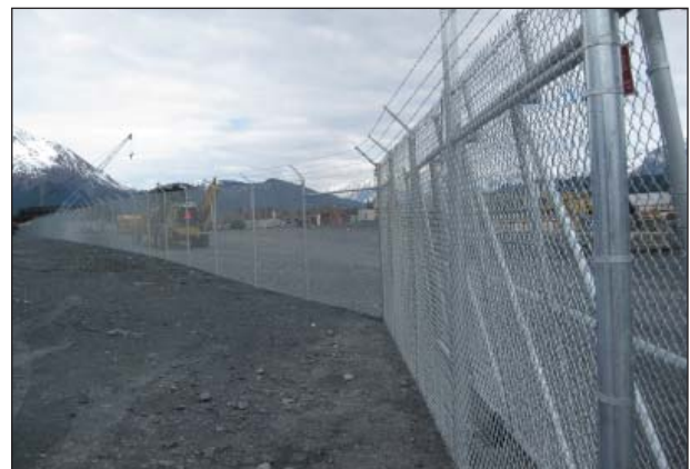
On the west side of the terminal, a new 6-foot fence will be erected and link to an existing fence along the East Dock.
