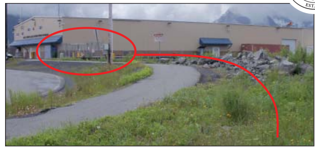
The existing gates on either side of the terminal will be replaced with automatic roller gates equipped with card reader controls. New 6-foot fencing will connect to the gates.
