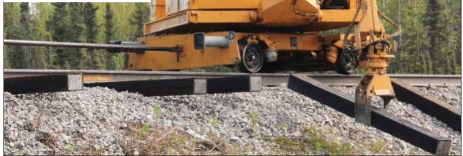
A tie crane operator positions a new tie during tie replacement operations in spring 2011. Inset: A track laborer replaces a missing spike on the track north of Wasilla.
