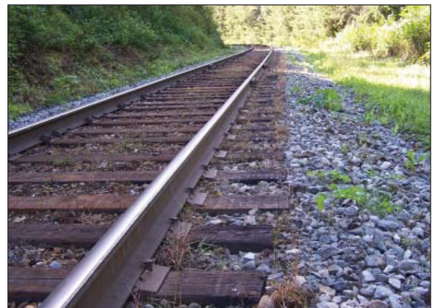
Post herbicide control near Seward. Note clear distinction at control area boundary at end of tie.
