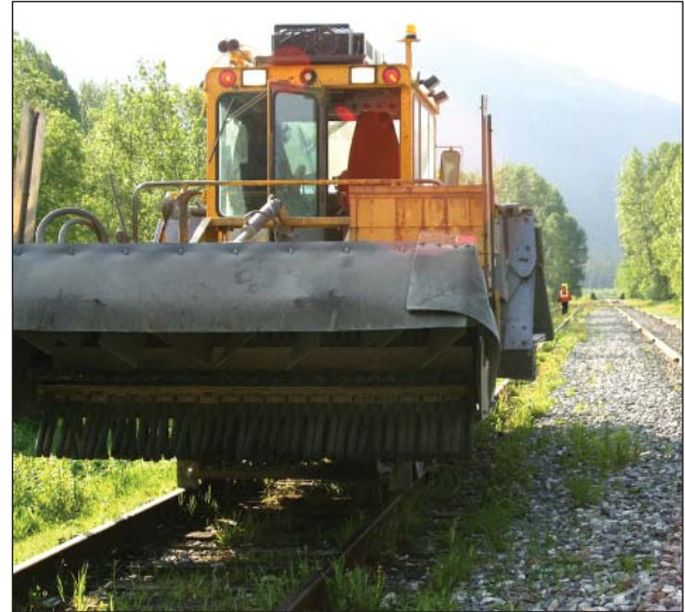
A ballast regulator is prepped to get to work on a stretch of track with significant vegetation coverage. The ballast regulator will turn over the track bed rock material (ballast), which hinders weed growth temporarily.
