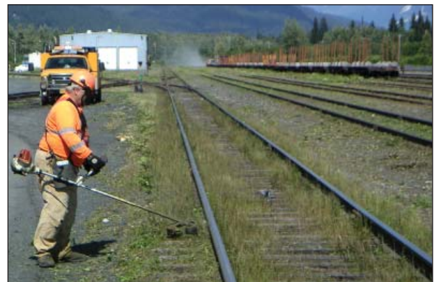
Ineffective mechanical/manual control in Seward yard prior to chemical application.
