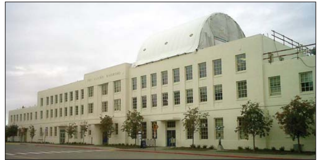
Phase 2a included installation of a paved-system roof along with more insulation for better energy conservation.
