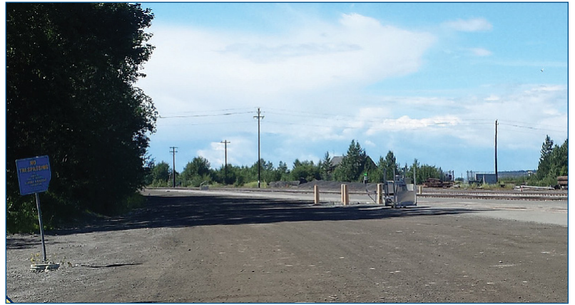
The project will improve the existing gravel access roadway running along the south side of the main line track.
