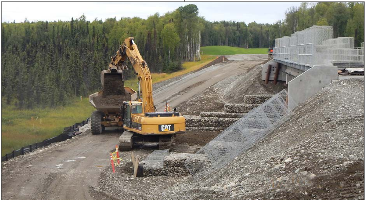
Segment 4: 2015 summer work on a 140-foot 5-span concrete girder bridge over a tributary to the Little Susitna River.
