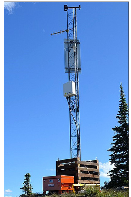
Example of Weather Monitoring Station
