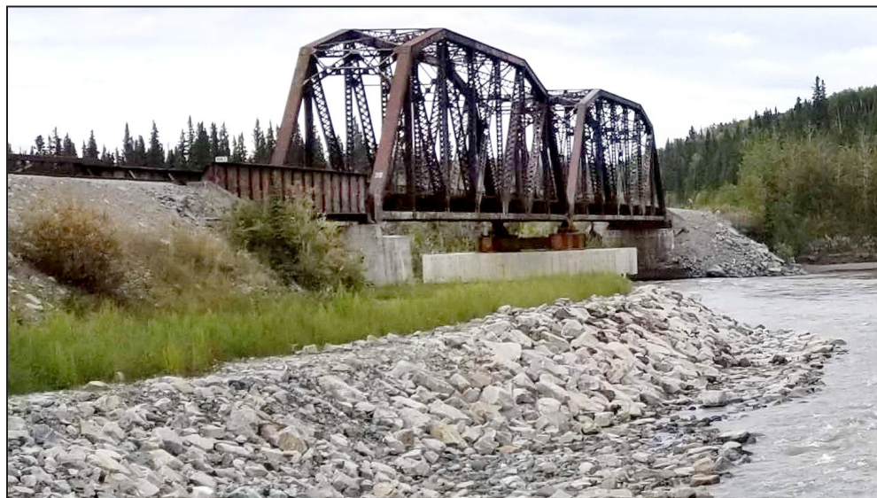
Bridge 370.7 crosses the Nenana River near the small, remote community of Ferry, Alaska.
