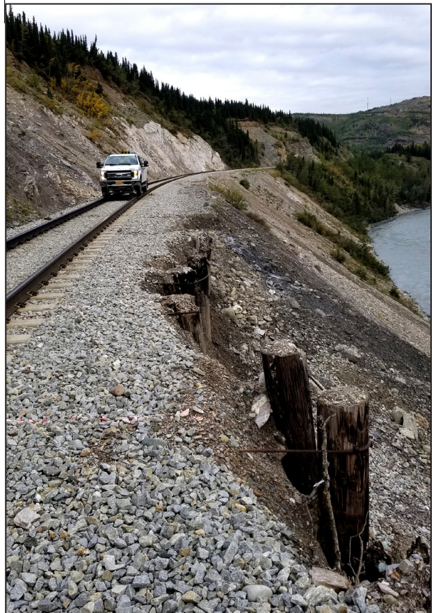
Several areas along the Healy Canyon corridor need to be stabilized to address erosion within the right-of-way.
