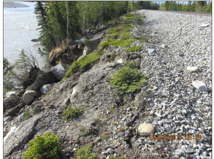
Railroad track embankment is eroding from Nenana River forces.
