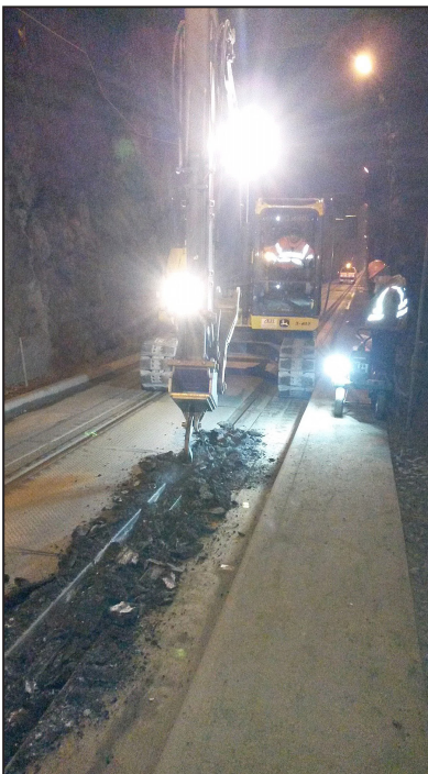
Above: Asphalt in the rail flangeways is broken up before removal. Right: Flangeways are cleaned before the rubber infill is installed, as depicted in the photo at far right.
