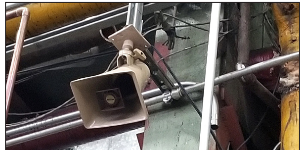
A mounted speaker that is part of the existing system, half of which is no longer functioning.
