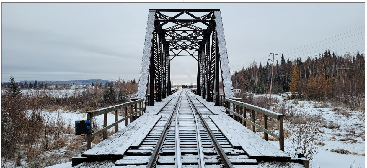
Bridge 467.9 crosses Noyes Slough, located just south of the Fairbanks Rail Yard.
