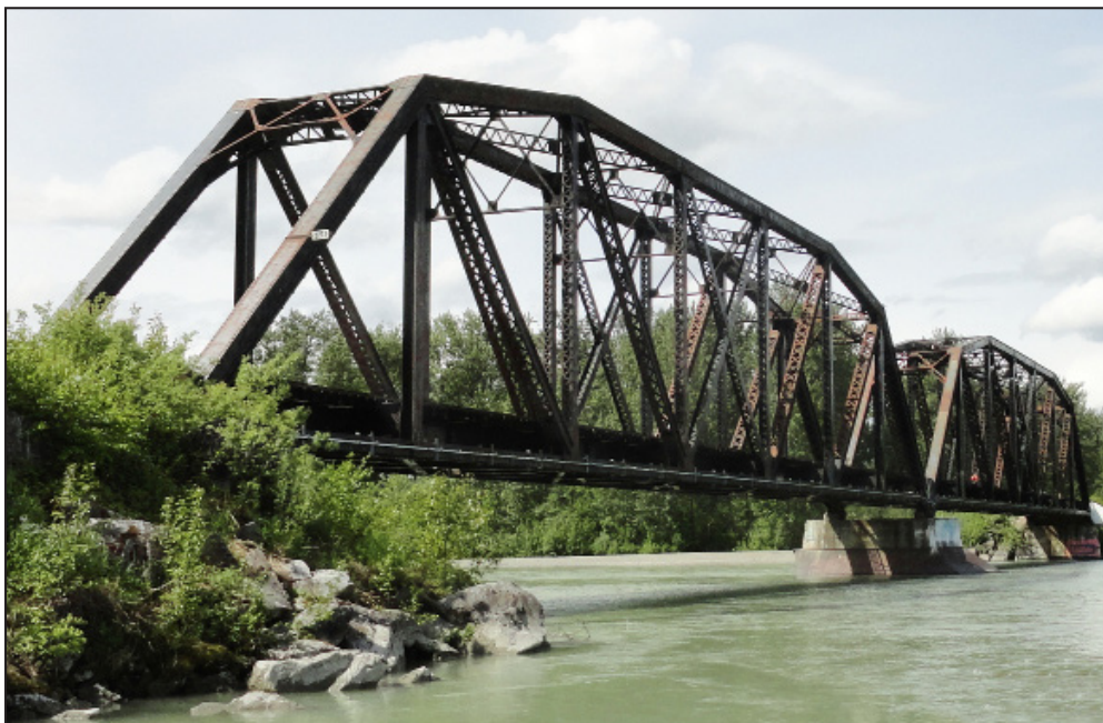
The 406-foot bridge features two steel through-truss spans that will be rehabilitated.
