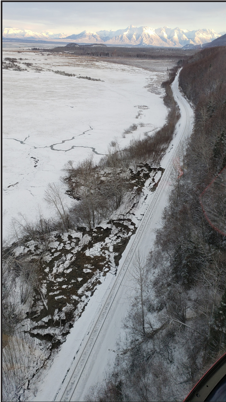
The 2018 earthquake caused shoulder and sub-structure damage along a stretch of track about 25 miles north of Anchorage.
