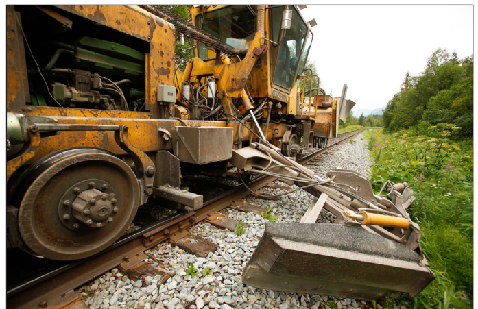
A ballast regulator is equipped to scrape weeds along the side of the track bed, which tempers weed growth temporarily.
