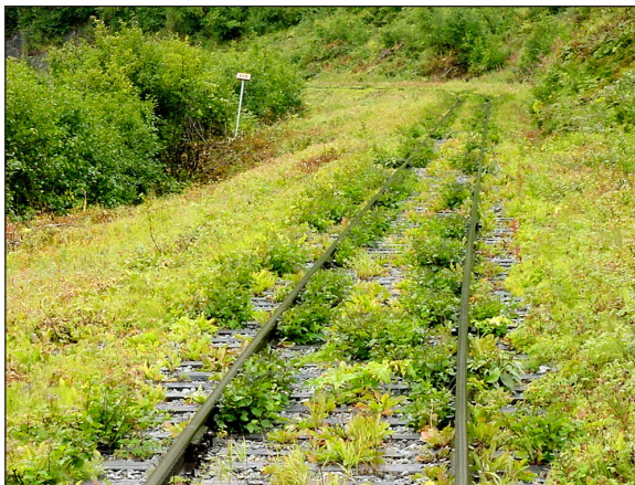
Overgrown weeds on the track are nearly impossible to eliminate with non-chemical methods.
