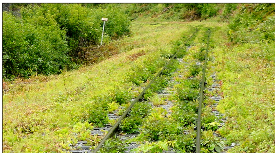
Overgrown vegetation poses many risks and dangers.
