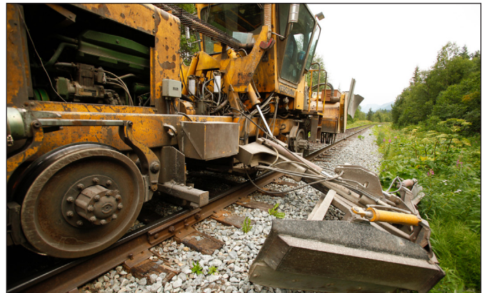
A ballast regulator is equipped to scrape weeds along the side of the track bed, which tempers weed growth temporarily.
