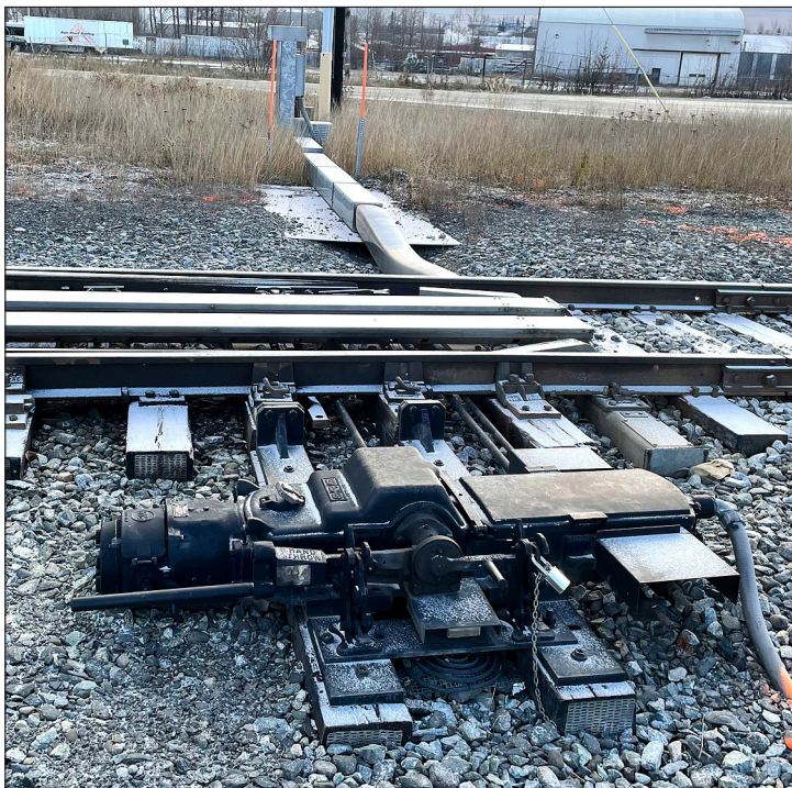
Aging powered switch machines like this one will be replaced.
