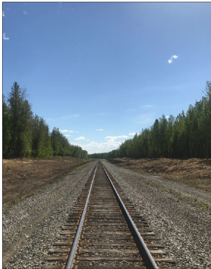
The stretch of Alaska Railroad right-of-way near Willow shows the results of clearing work.
