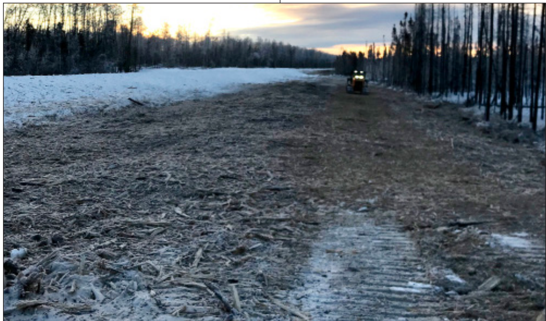
Taken in February of 2020, this image shows clearing activity during the winter. Ash is still visible in the mulch debris due to the scorched and burned trees left standing after the 2019 McKinley fire.
