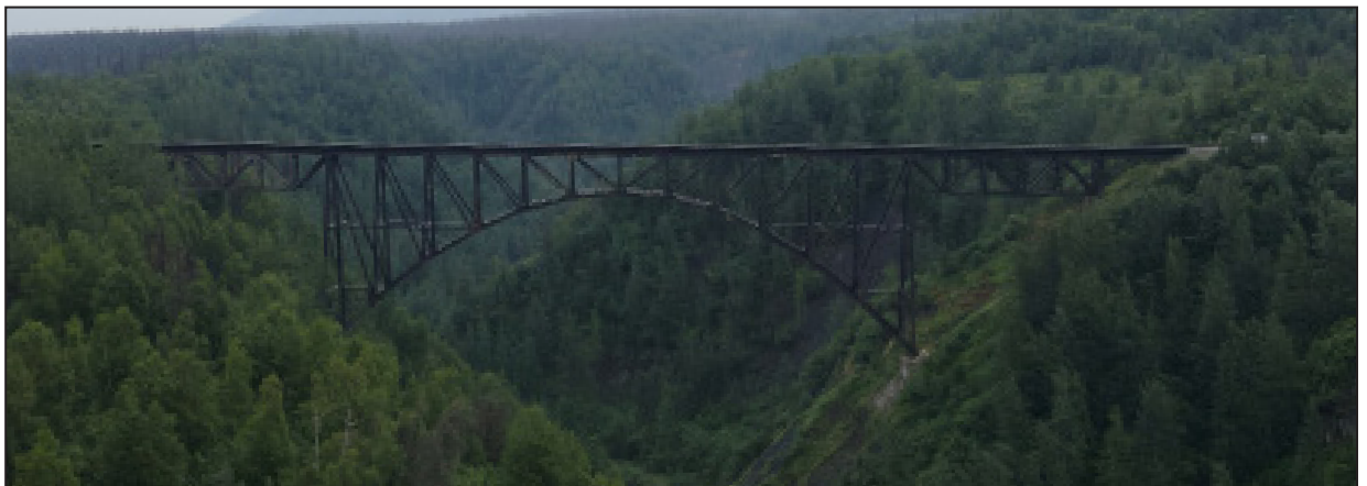
The 914-foot steel bridge spans Hurricane Gulch at ARRC milepost 284.2, about 60 miles south of Denali.
