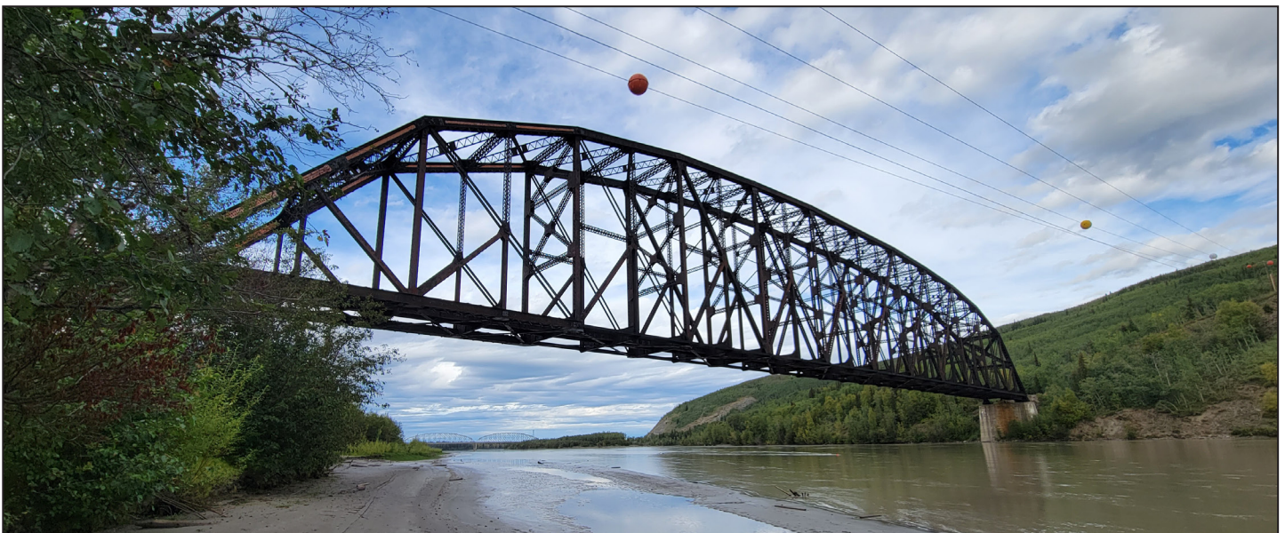
East view of bridge 413.7, the bridge's top chord will be rehabilitated, as well as hangers and interior floor beams.
