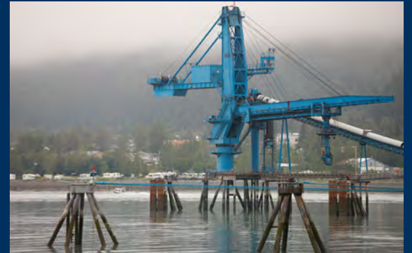
Photo III-1.13: SLF Dock with Conveyer and Ship Loader (Source: Judy Patrick Photography, 2012)
