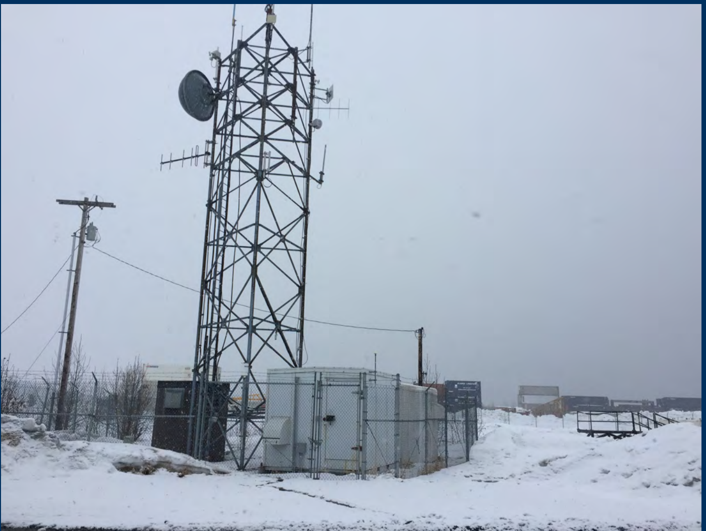
Photo IV-4.5: Existing Communications Tower and Equipment in Freight Yard (Source: DOWL, 2017)
