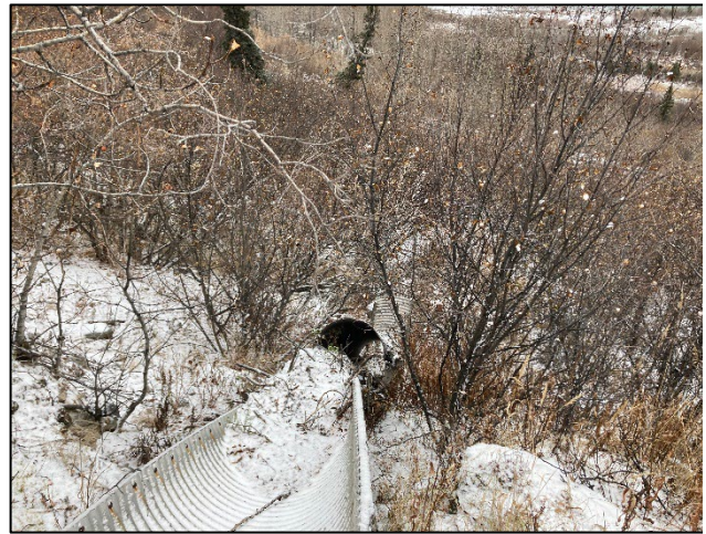
Photo 2.2: Section of disconnected pipe in the Middle Flume, looking north
