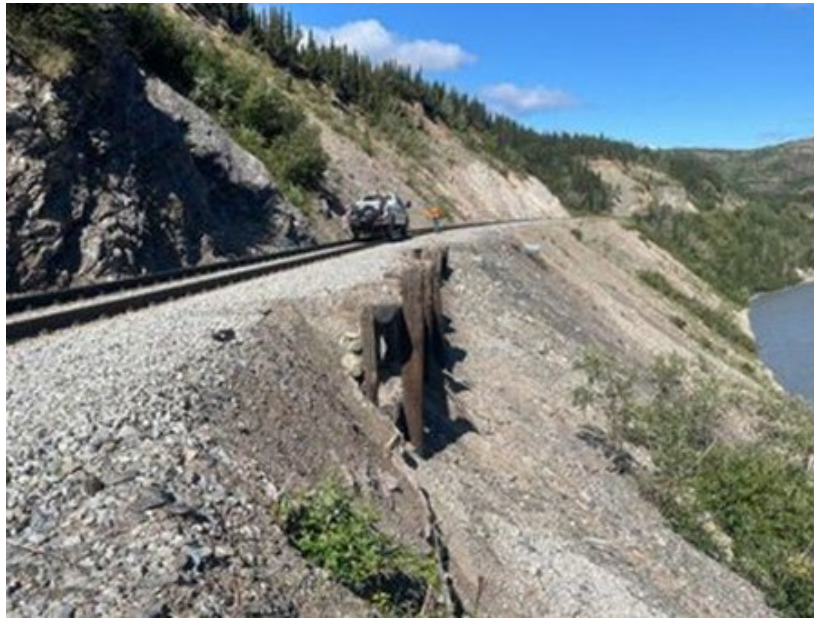
Figure 2-7: Wall # 41 - condition rating: poor
