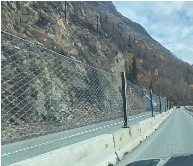
Figure 2-6: Jersey barrier enhanced with fencing
