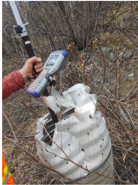
Figure 2-9: Vertical 12-inch CMP rated in poor condition at MP353.48
