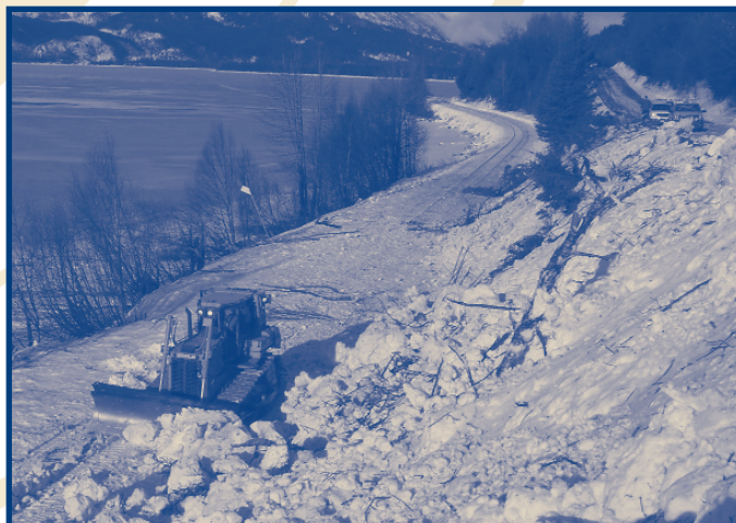
Rail and road crews work to clear the debris from a snow slide in February.
