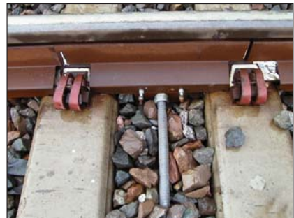
System gauges and cables are installed under a protective rail covering that attaches to cable conduit.
