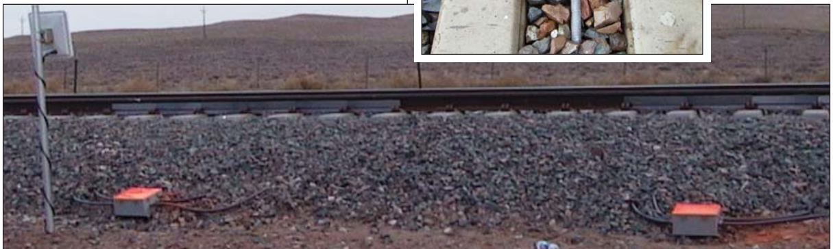
The WILD strain gauge and cables are installed along the rail, with cable conduit leading to track-side junction boxes and system electronics.
