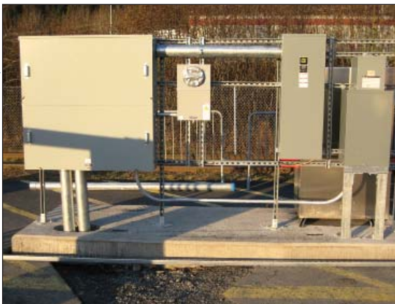
A new shore power cabinet system is installed nearby the Depot in Seward.
