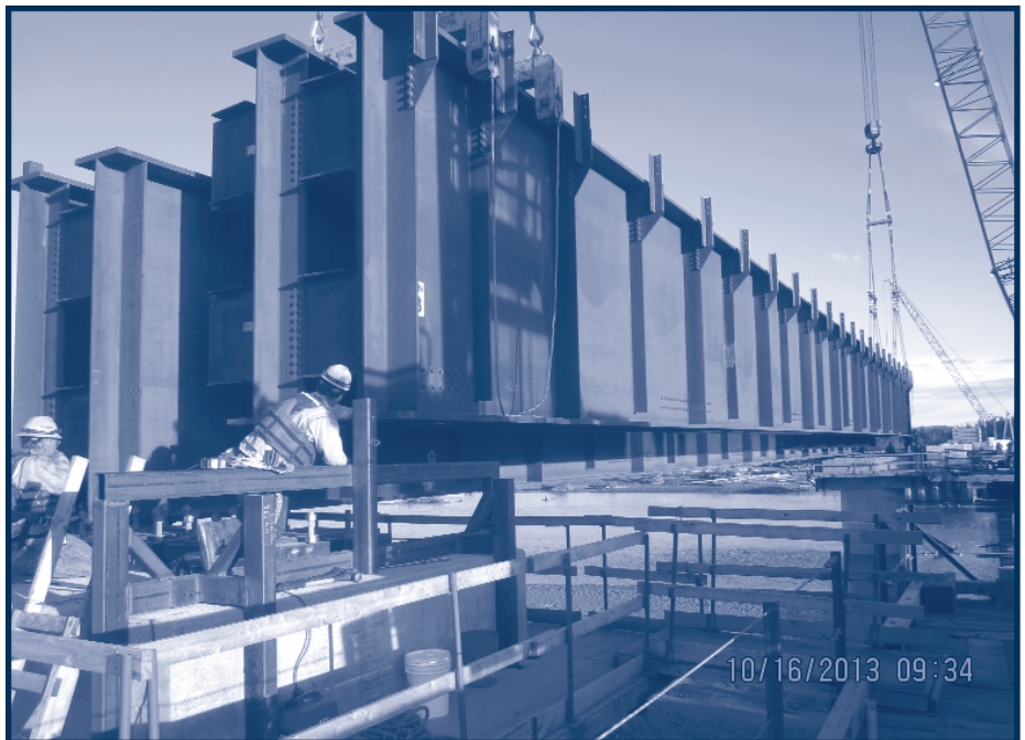
The first steel girder is set upon piers 6 and 7 in October 2013. Since then progress continues at a good speed to keep the project on target for completion in July 2014.
