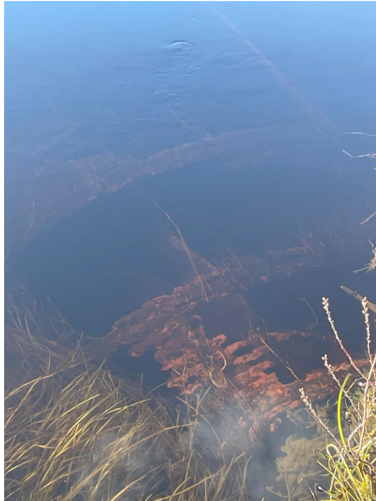
Photo 3. MP 66.09 culvert outlet (submerged).
