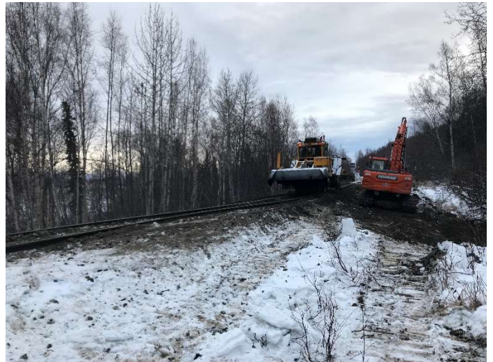
Photo 4: The BR20 and the DX180LC working at the ≈MP 138.5 worksite, looking RR North.
